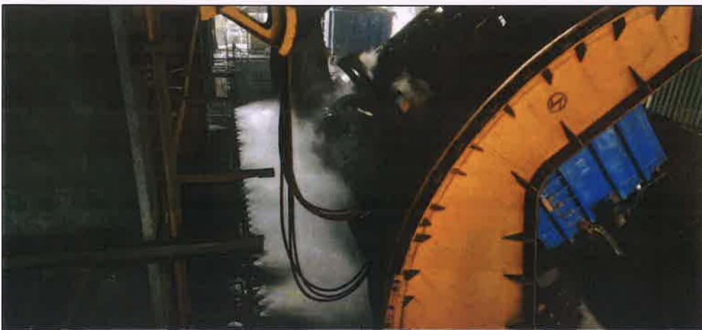
Fig.2: Water fogging system at wagon tippler.
