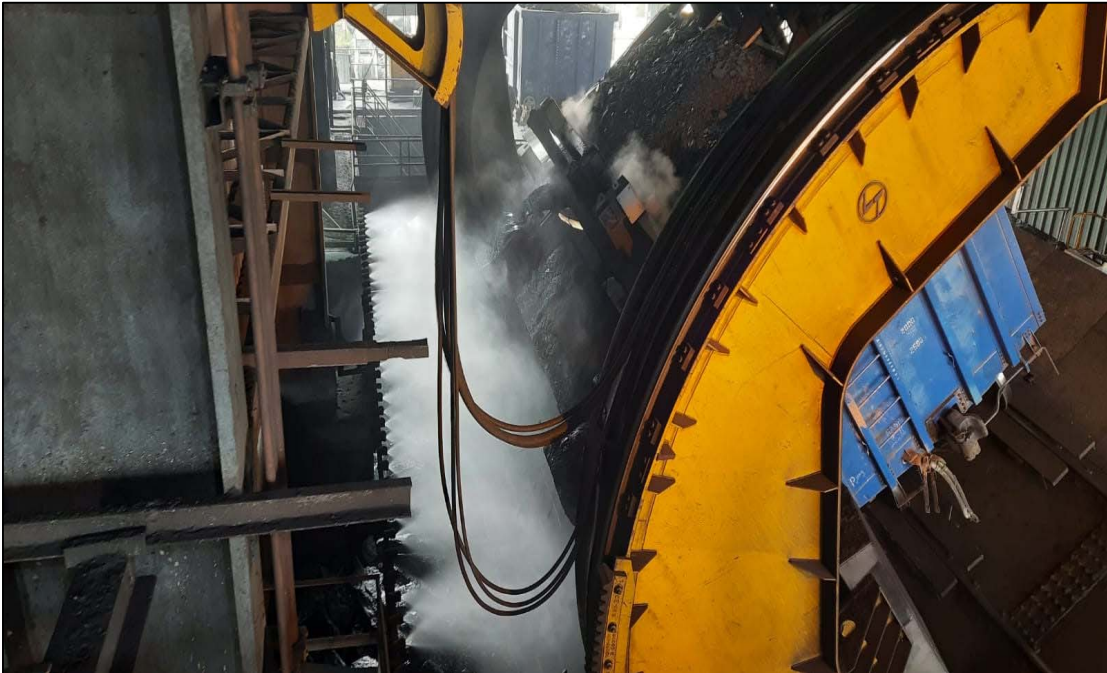
Water fogging system at wagon tippler.
